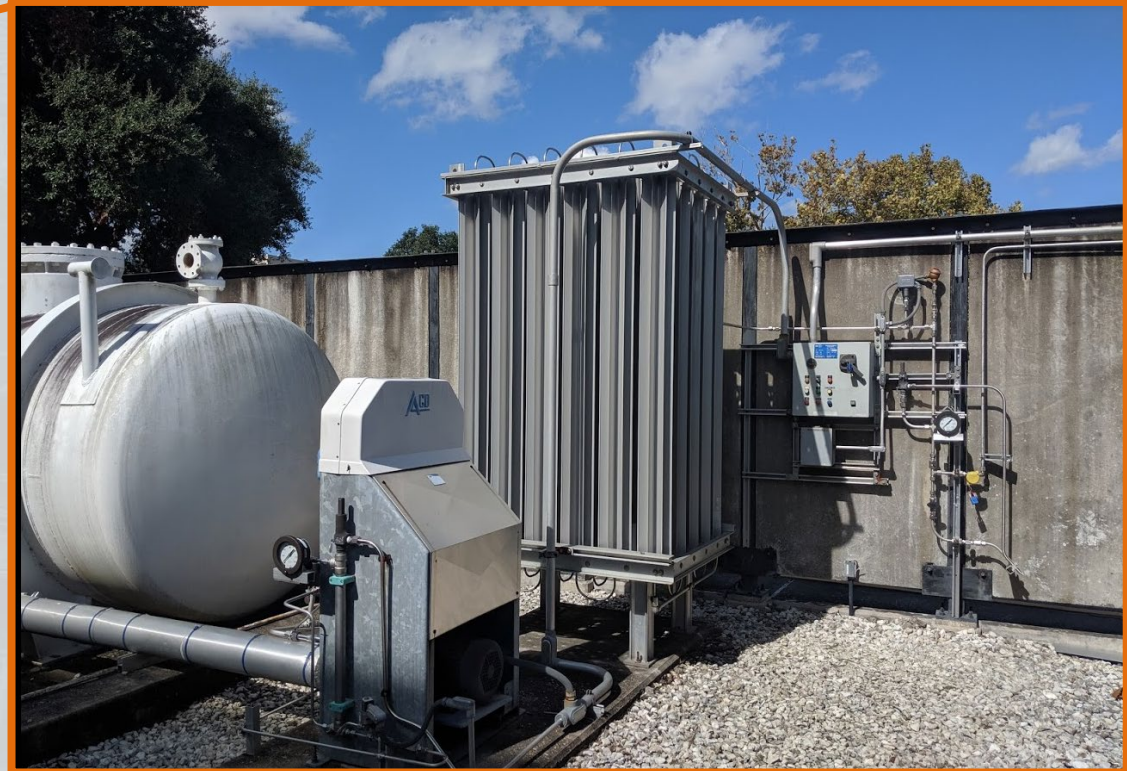
LN2 tank, pump, and ambient vaporizer
