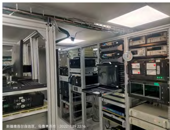
Fig. 3 The digital backend systems for VLBI and single dish operations, working in the walk-in electromagnetic shielding box under the telescope base.
