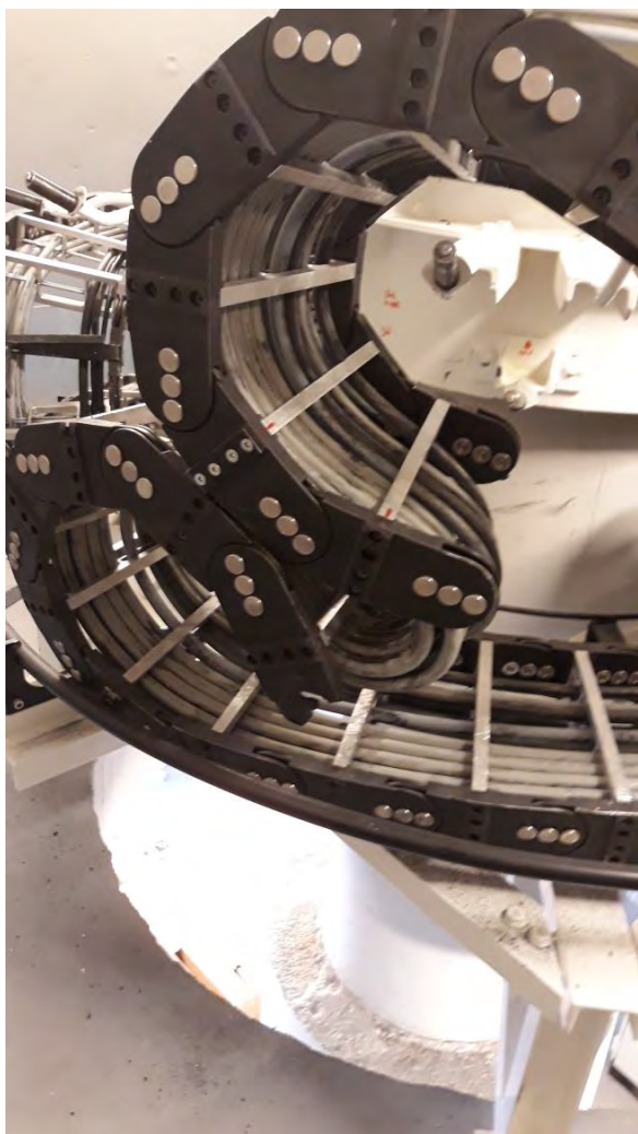
Fig. 3 Detail of the cable wrap structure breakage.
