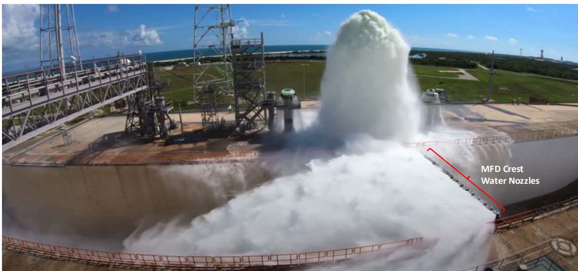
Fig. 3 Water injected from the MFD crest at LC-39B during a water system flow test.
