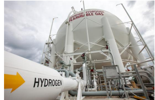
LH2 Storage Tank and transfer line at NASA's KSC
