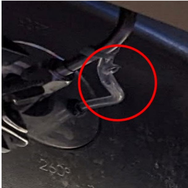
Tygon tubing - area circled shows blistering on the FOSS repressurization line
