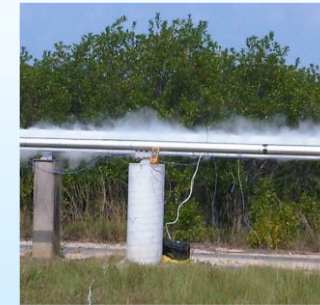
Cryogenic Fuel Line Monitoring
