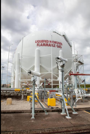
LH2 Tank at Pad 39B
