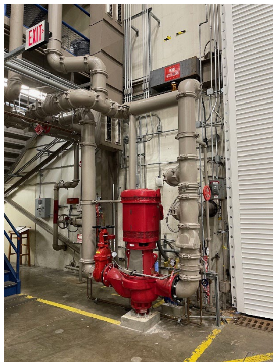
Figure 2. JSC Building 7 Fire Booster Pump
