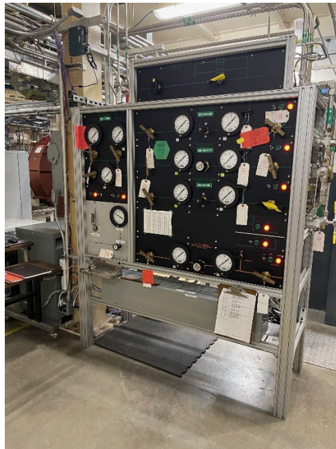
Figure 4. 20 FT Oxygen Panel
