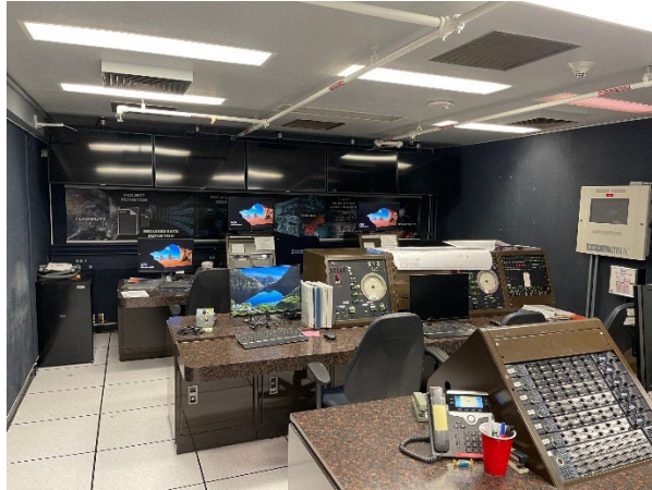
Figure 6. 20 FT Control Room
