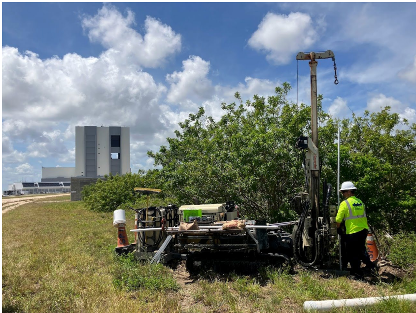
Photo of driller installing MW screen. Vehicle Assembly Building (VAB) pictured in background.
