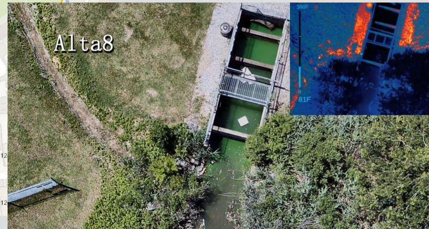
North Marvin Storm Drain Outfall Inspection with IR
