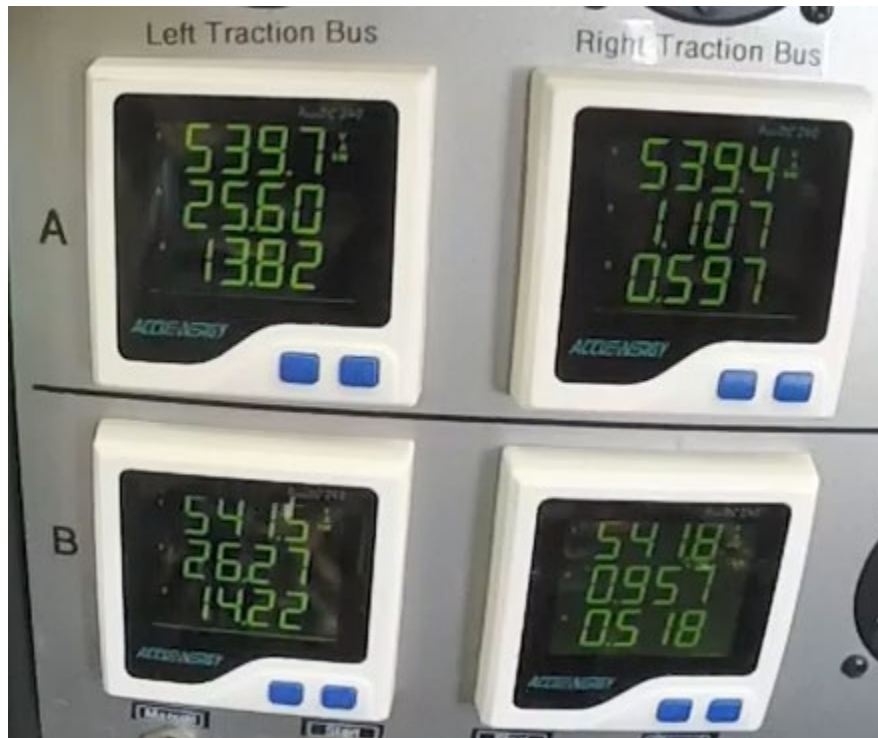
Fig. 9. Traction bus energy meters displaying from top to bottom: voltage, current, power.
