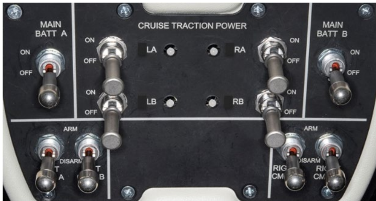
Fig. 6. High voltage switches.
