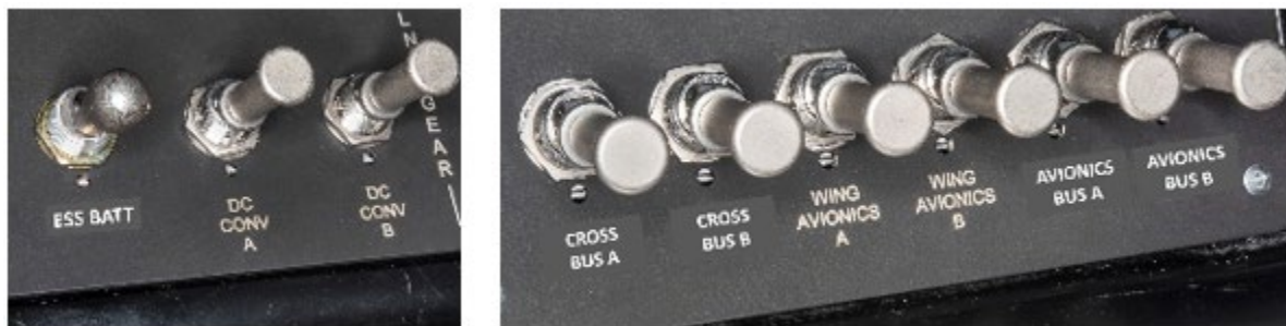
Fig. 5 Low voltage switches.
