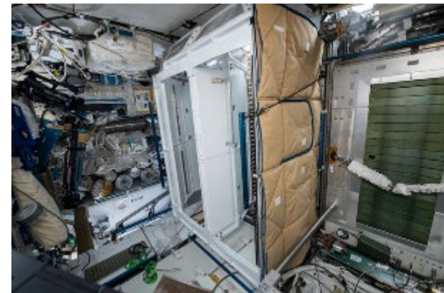
Toilet Integration Hardware Stall installed in Node 3, ISS
