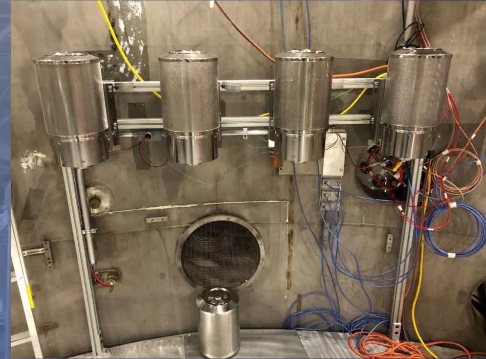
20 FT Air Revitalization System, 1 st Floor
