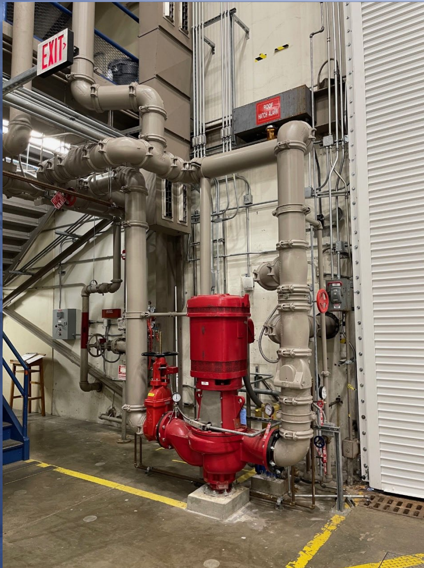
JSC Building 7 Fire Booster Pump
