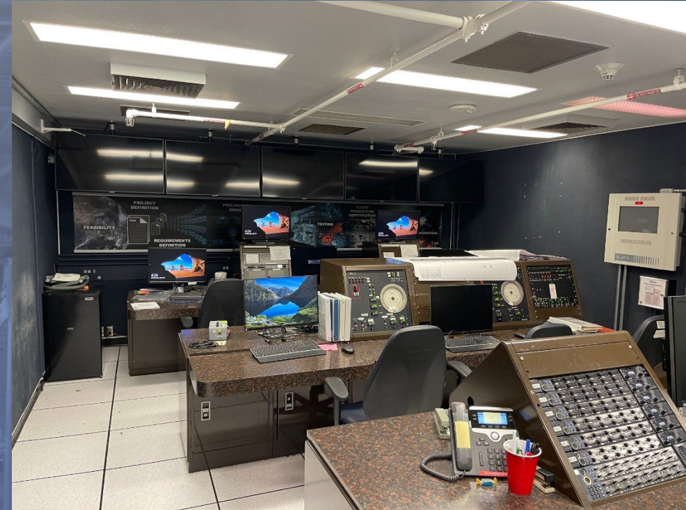
20 FT Control Room
