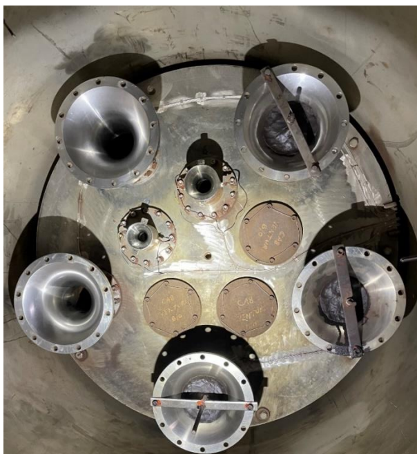
Figure 40: Main Airflow Choked Flow Venturis
