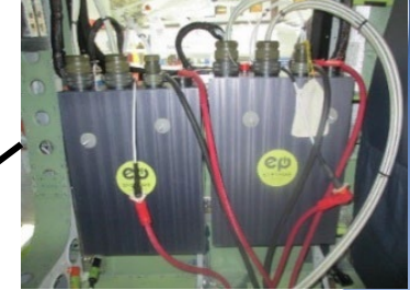
Battery Control Module
