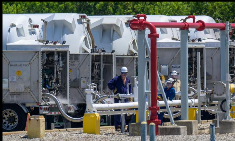
Tanker trucks replenish liquid hydrogen (LH 2 ) within large sphere at NASA's Kennedy Space Center in Florida, Launch Pad 39B. (NASA Image NHQ202208310013)
