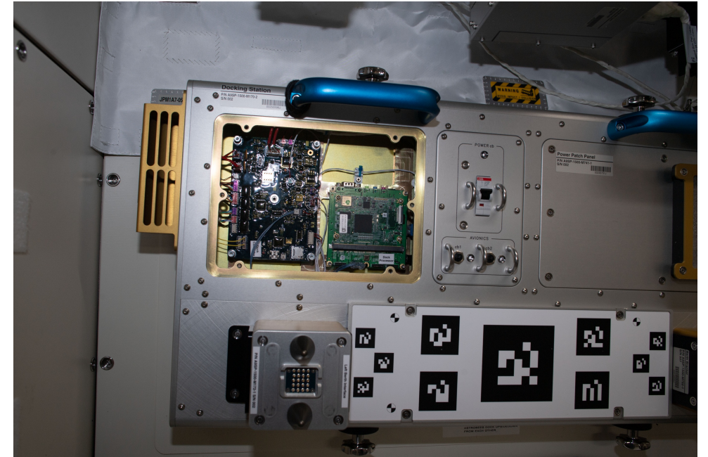
Dock's avionics patch panel removed
