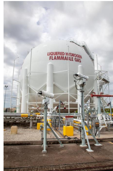
800,000 gal (3,3028 m 3 ) LH2 Tank at Pad 39B
