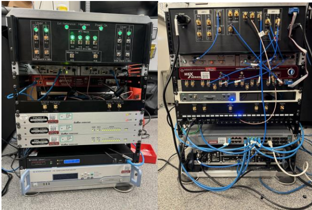
Figure 22. RF rack (partially wired) front and back
