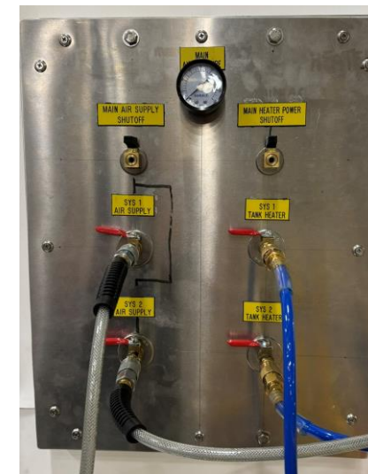
Notional Tank Utility Control Panel on Habitat
