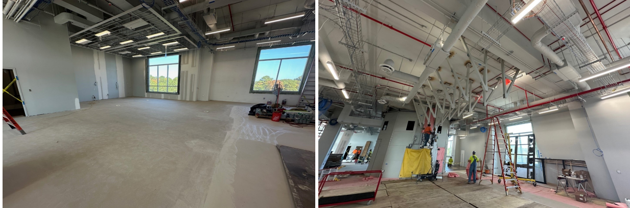
(a) Control room
