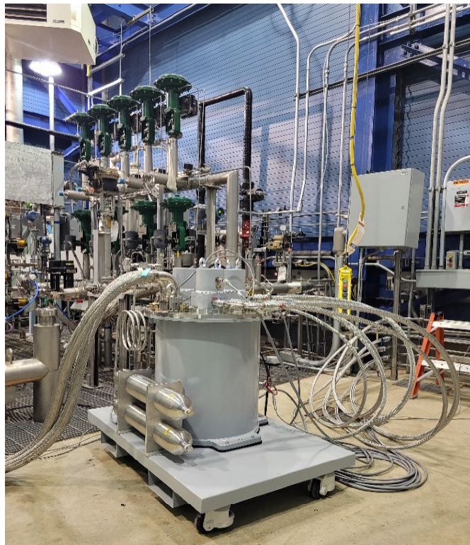
Figure 9.—Cryocooler assembly connected to facility.
