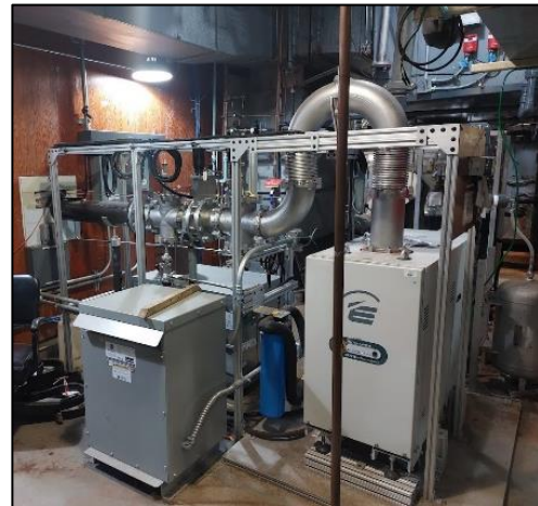
b) Vacuum Pump System
