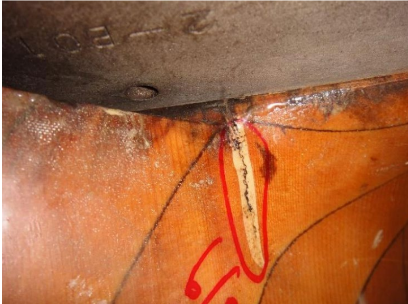
Crack found during 2018 inspection
