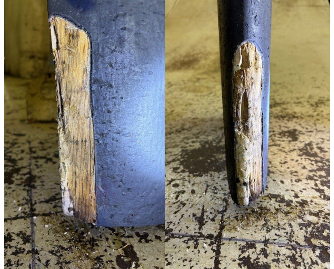
Leading Edge Damage 2024
