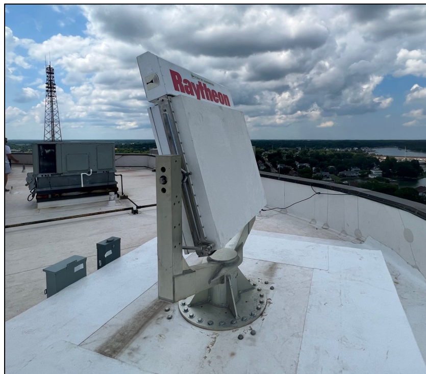
Figure 1-13. Skyler-2 Radar Installed Atop Hampton Harbour Centre
