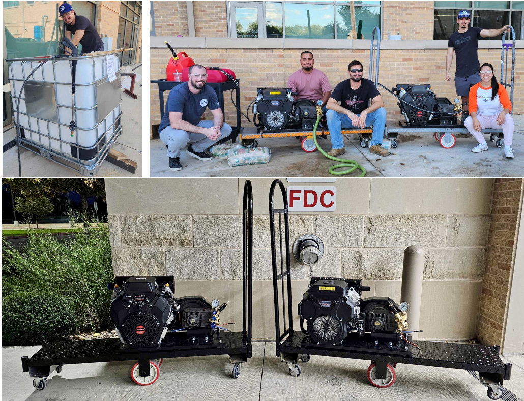
Fig. 21 Coolant flow infrastructure, including water storage ( left ) and gasoline-powered pumps mounted on mobile carts ( right ).
