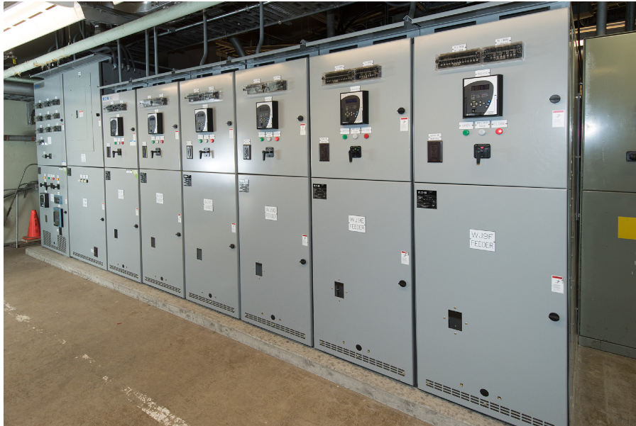
Figure 23.—PSL main 2,400-VAC switchgear. (C-2014-08192)
