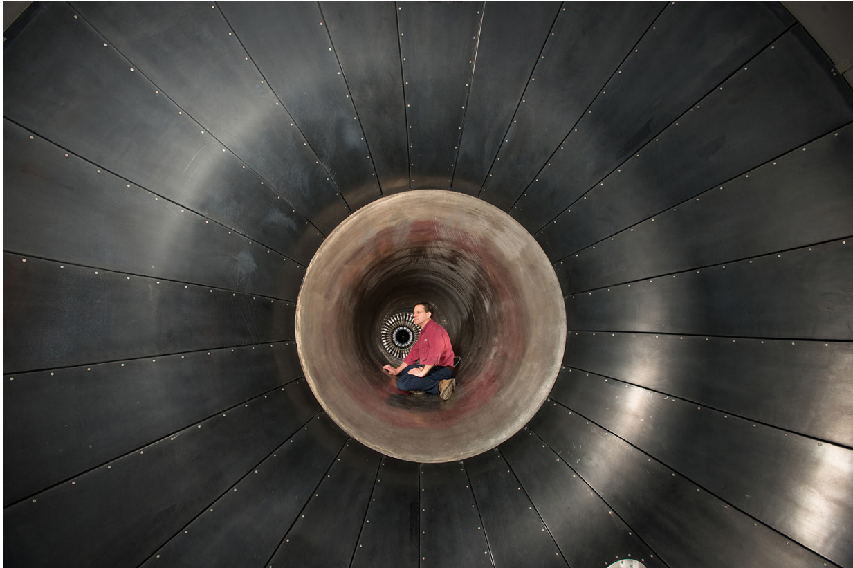
Figure 34.—Carbon fiber transition duct mounted in PSL-3 inlet plenum.
