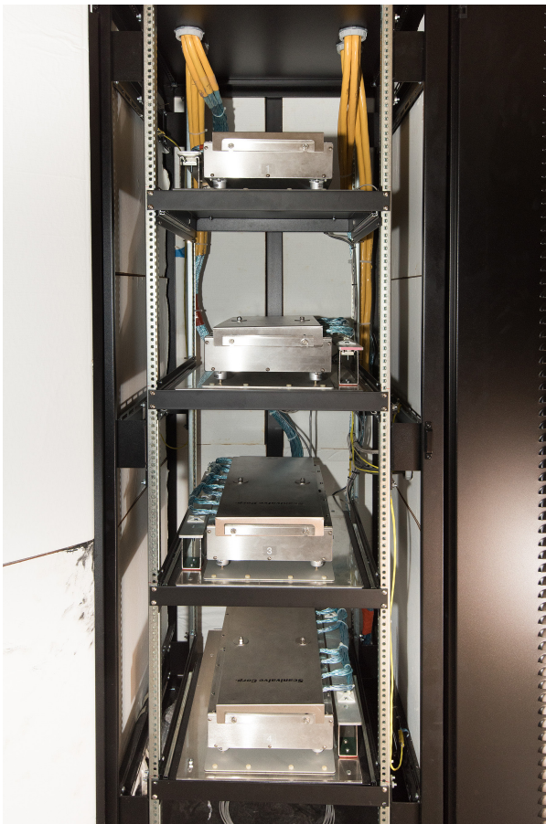
Figure 36.—Typical Scanivalve DTS equipment rack. (C-2014-08134)
