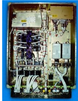
Main Bus Switching Unit
