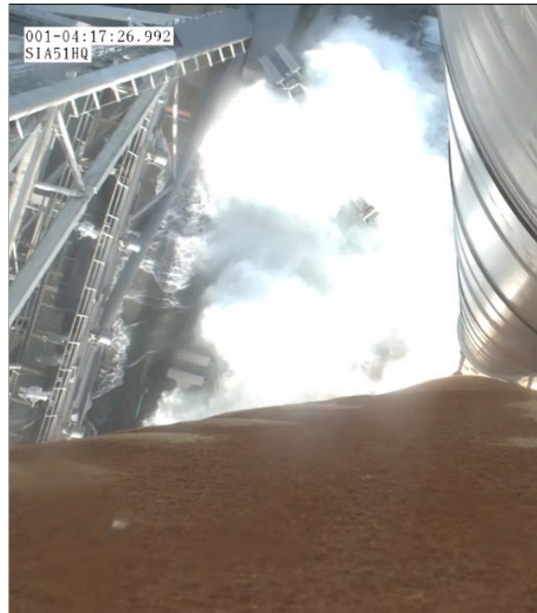
Figure 4 Water Suppression System (Full Flow)
