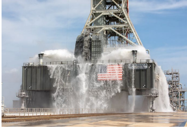
Figure 2 Water Suppression System 2
