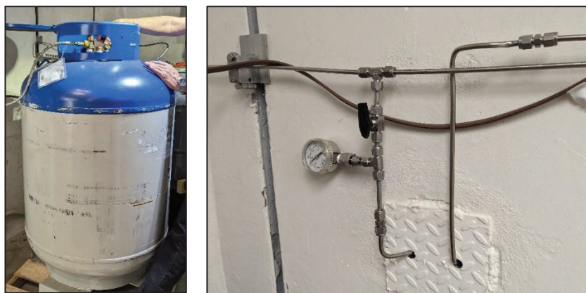
Figure 2. Solstice PF 1,000-lb cylinder (left) and in-lab plumbing for fluid use (right)
