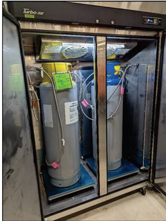
Figure 4. Clean (Right, Blue) and Dirty/Collection (Left, Yellow) Solstice cylinders in refrigeration unit at MAF Cleaning Facility
