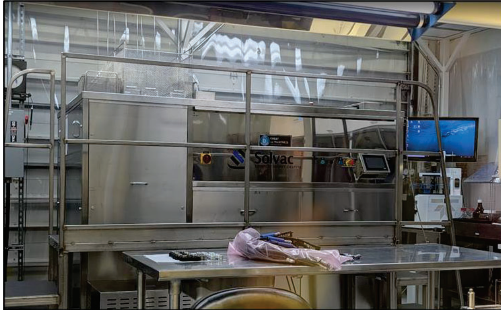
Figure 10. NBL Vapor Degreasing System
