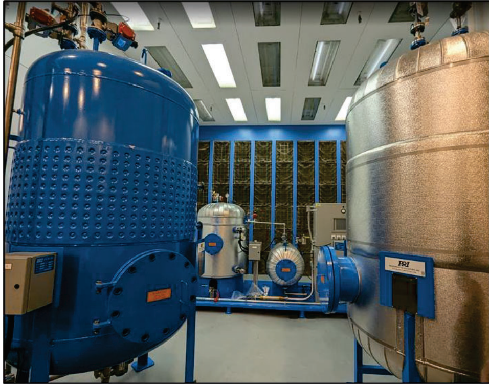
Figure 9. JSC New Solvent Distillation System
