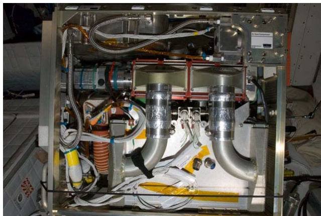
Figure 2. Amine Swingbed installed inside the double locker.
